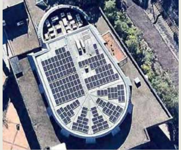
Aerial photo after solar installation
