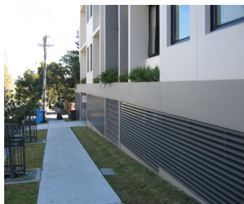
Figure 22.3-2: Ventilation grilles to basement car park are well integrated with overall facade design.
